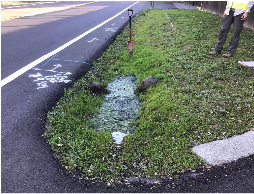
Photo 17. Sample Point 6 (SP06). Sample point located in the lowest point in a roadside ditch. A blocked culvert adjacent to the ditch could be causing the recent ponding.
