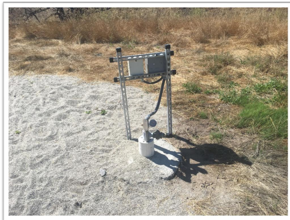
Photo 2: Alternate view of Project well. Installed to 300 feet with 100' annular seal.
