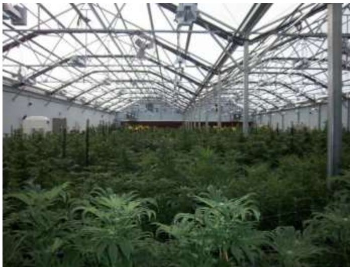
View of greenhouse structure and equipment to show need for maintenance
