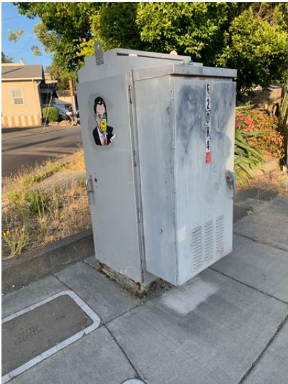
Utility Box on the corner of Mountain Avenue and Highway 12.
