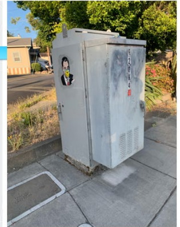
Utility Box on the corner of Mountain Avenue and Highway 12.
