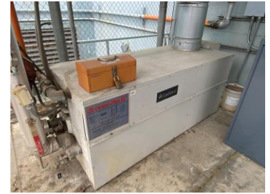
Existing auditorium hydronic boiler
