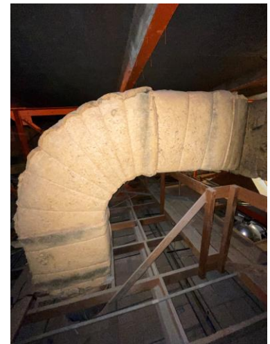
Ductwork serving auditorium
