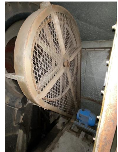
Existing auditorium air handler
