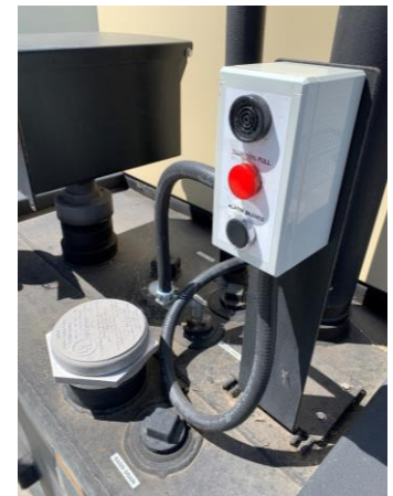
Generator fuel shutoff alarm
