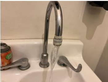
Sink missing aerator and no faucet controls
