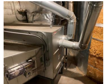
Existing Club Room furnace
