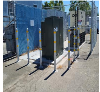
Existing transformer, generator, and main service board
