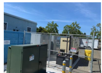
Step down transformer, generator, and main switchgear
