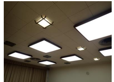
North Room lighting
