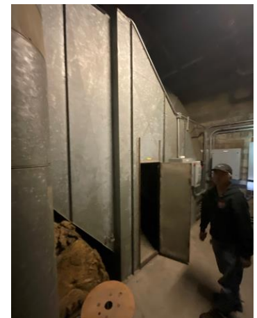
Existing air handler serving auditorium
