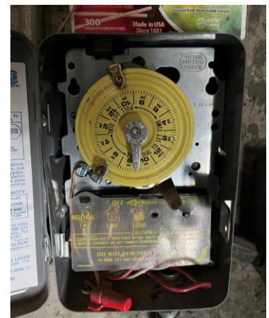
Timeclock controlled recirculation pump
