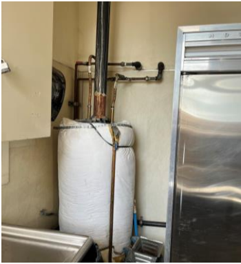
Club Room water heater
