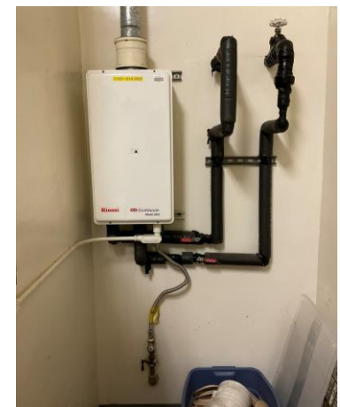
Tankless water heater serving commercial kitchen
