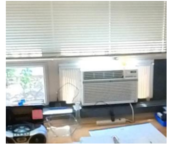
Existing office window A/C unit
