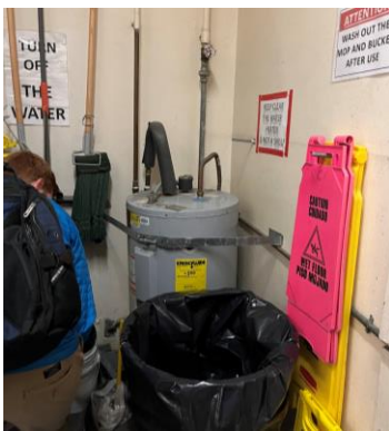
Janitor closet water heater
