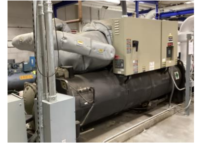
Existing chiller at CMP
