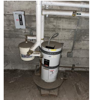
Existing electric resistance water heater to remain
