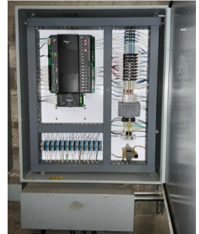
Existing Andover Control system for HVAC control
