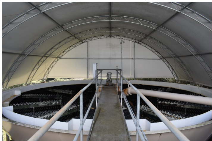
SDC Water Treatment Plant
