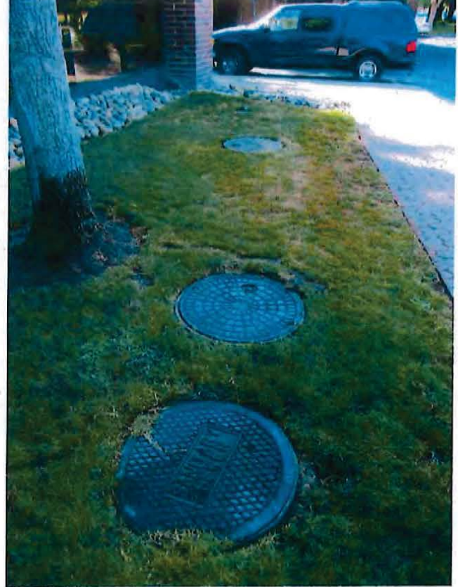
8. Grease interceptor at 2235 Challenger Way.
