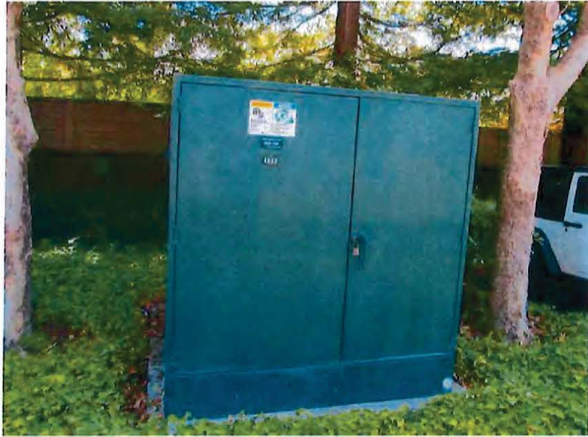
33. Pad-mounted electrical transformer.
