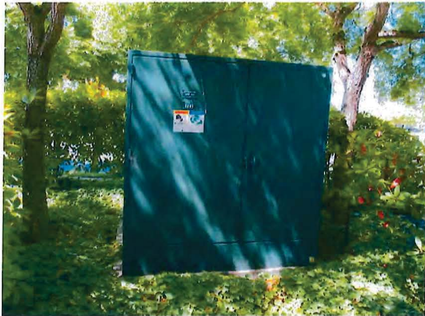
34. Pad-mounted electrical transformer.
