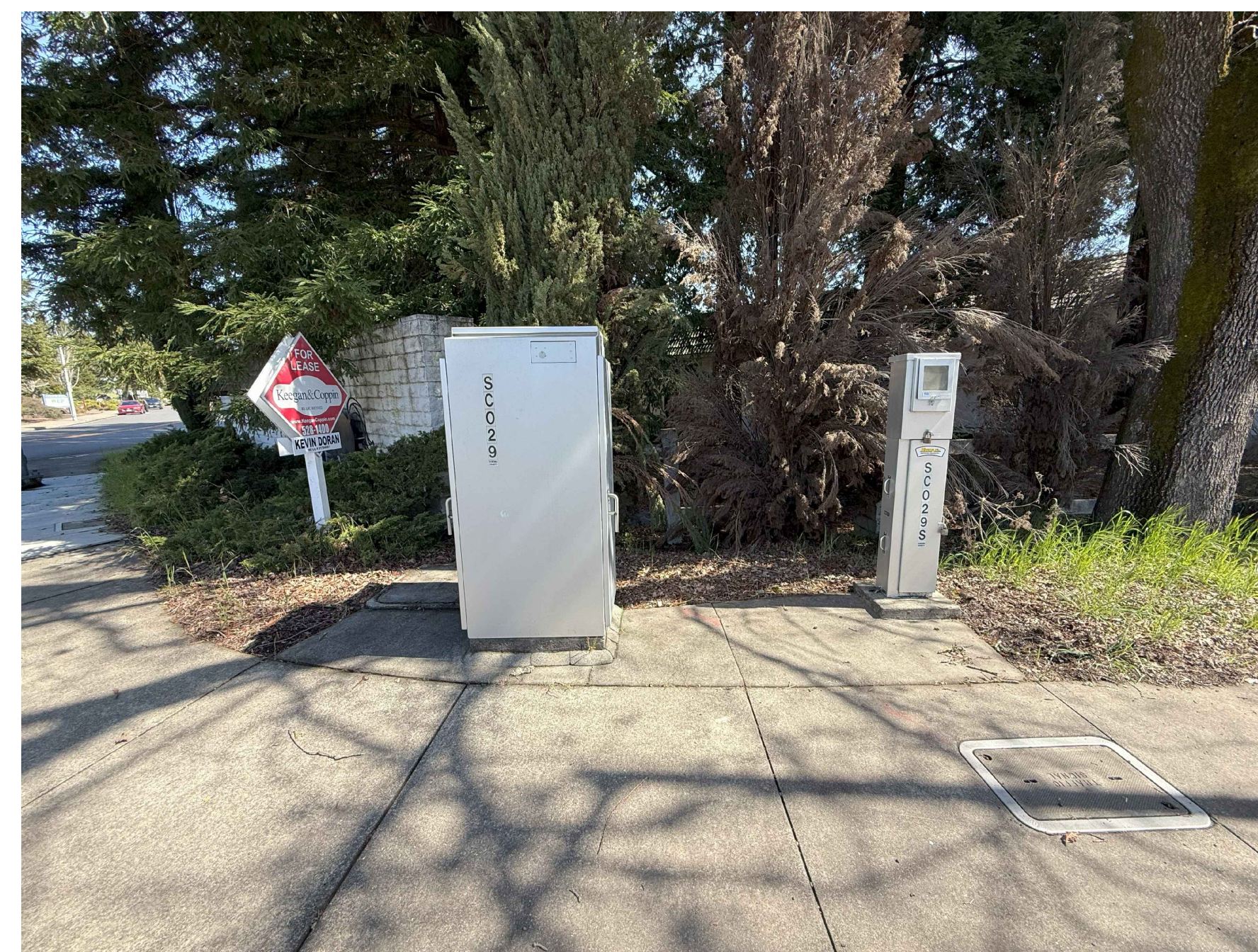
WIKIUP DR X OLD REDWOOD HWY - CONTROLLER CABINET
