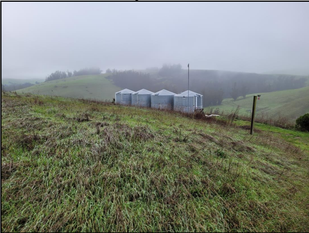
Photo 6: View of four (4) steel water tanks used to store water from the irrigation well.
