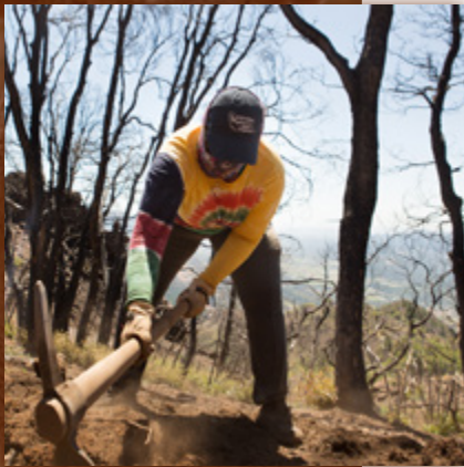
Trail work on Hood Mountain Regional Park and Open Space Preserve is underway.
